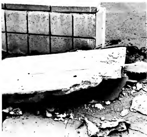
Photo 13. About 27 inches of sidewalk overriding in front of one of the buildings shown in photo 12 indicates the local extent of ground surface shortening. E. G. Zacher photo.
